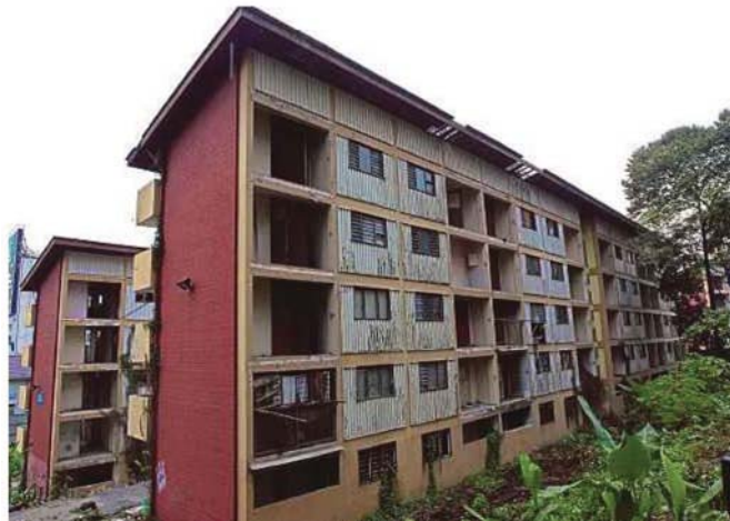
Residents of Block F of Taman Keramat Permai flats in Ampang Jaya, Selangor, were evacuated following the discovery of cracks at the block on Friday. PIC BY ASYRAF HAMZAH
